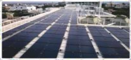
150kW PROJECT Bangalore, India
