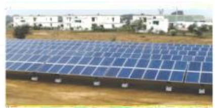
2.5MW PROJECT Rajasthan, India
