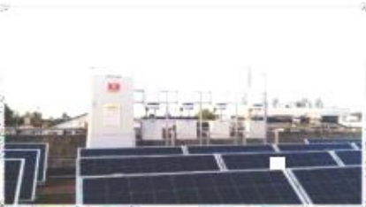
400kW PROJECT Tamil Nadu, India
