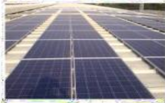
350kW PROJECT Tamil Nadu, India
